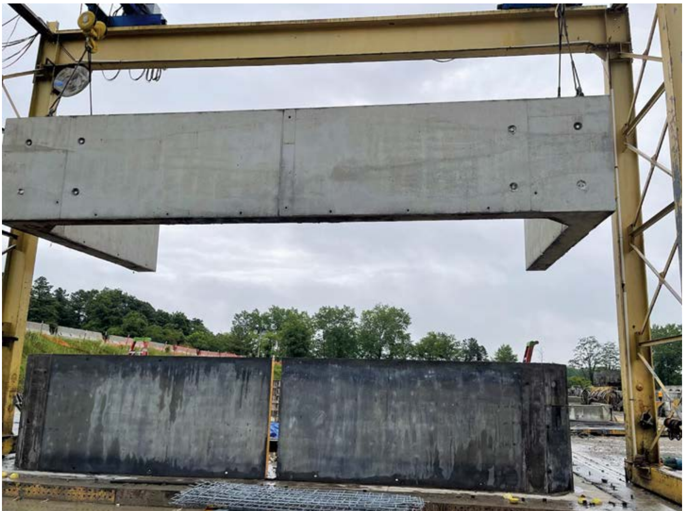
A culvert section is removed from its formwork and lifted by a crane at Garden State. Production for this project is taking place outdoors due to the size and weight of the culvert sections.
