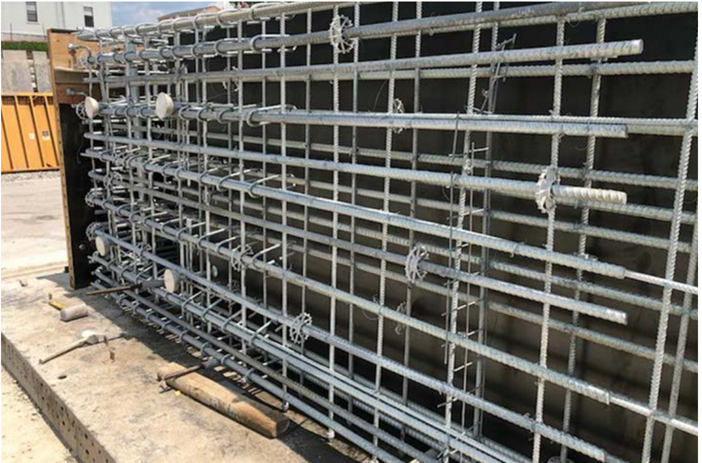
The precast concrete culverts are reinforced with 1 1/8-inch diameter (No. 9) steel reinforcing bars spaced every 6 inches. The design also uses stirrup reinforcement to increase the culvert sections' shear capacity.
